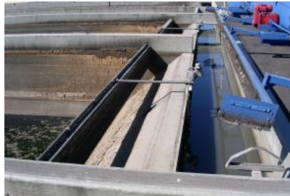
Hydraulic bottleneck: the primary clarifier
